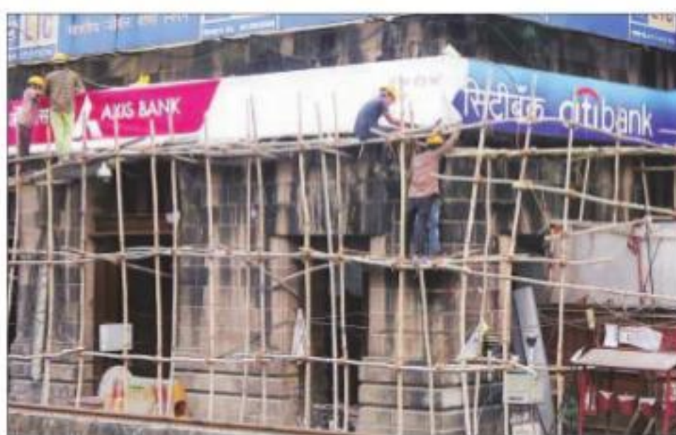
The signboard of Citibank being removed from the Mumbai office as part of the rebranding exercise with Axis Bank
