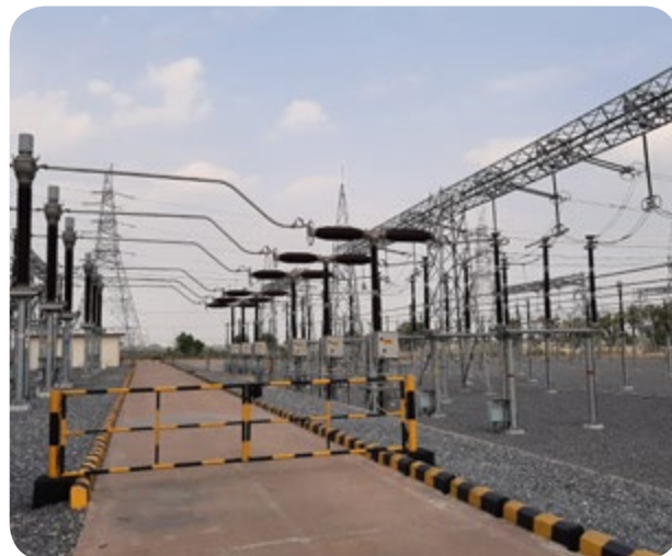
400 kV Air Insulated Substation for Odisha Power Transmission Corporation Limited (OPTCL) at Lapanga, Odisha
