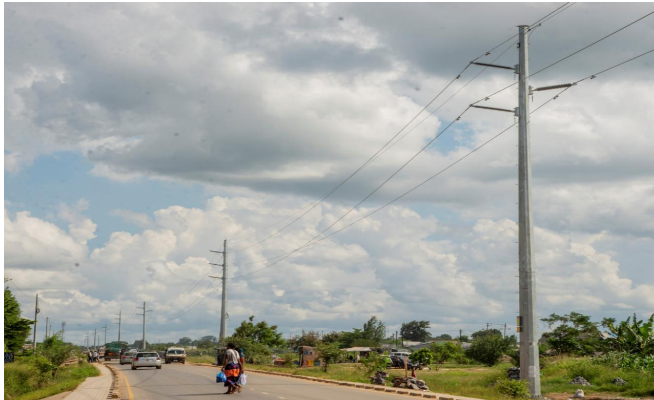
Construction of 132kV Single Circuit Transmission Line from Coventry – Waterworks, Coventry – Jimmy – Chawama for ZESCO in Lusaka
