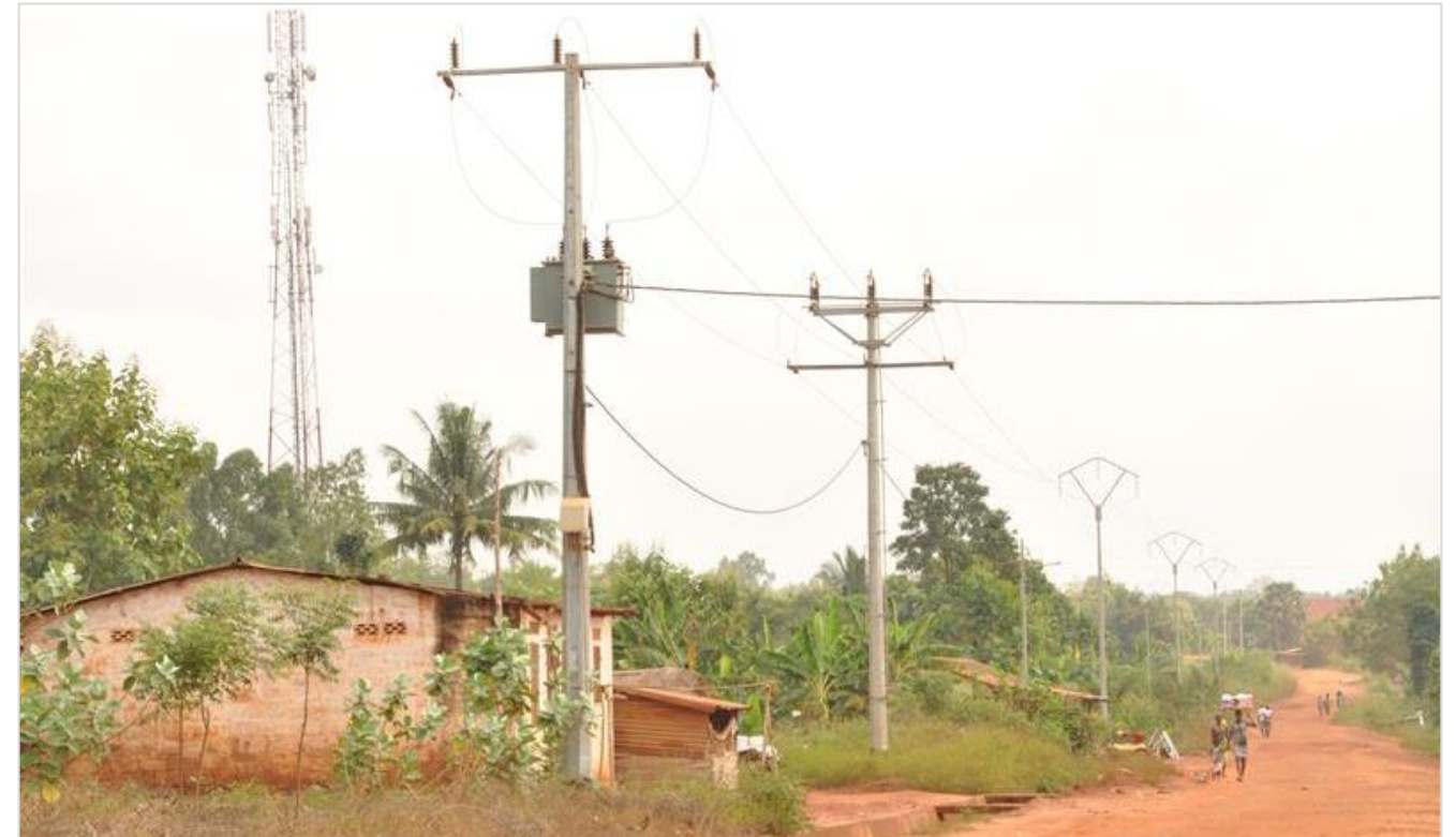
Medium and Low Voltage Networks for Rural Electrification of 46 Villages for Compagnie Energie Electrique du Togo (CEET)
