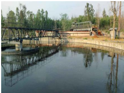
Secondary Clarifier - Pulp
