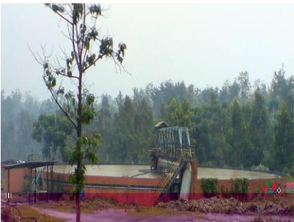
Primary Clarifier - Pulp
