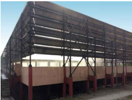
Mist Cooling System
