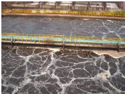
Diffused Aeration System
