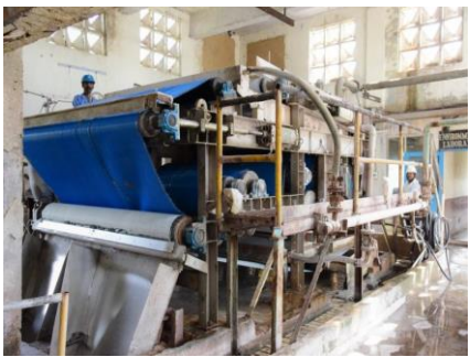
Sludge Handling - Paper
