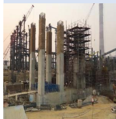
Unit #3 - Turbine Generator Deck
