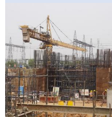
Unit #3 - Turbine Generator Deck
