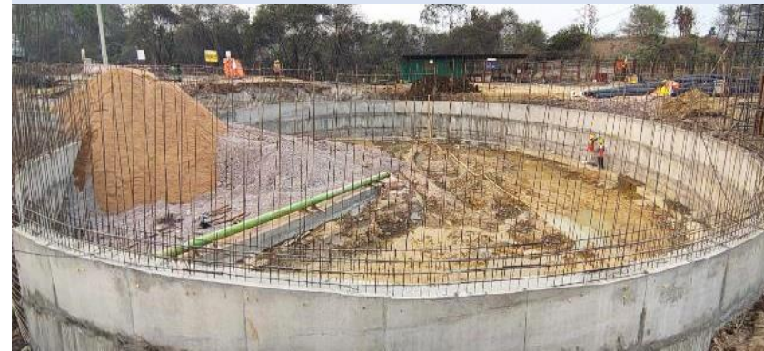
High-Rate Solid Contact Clarifier
