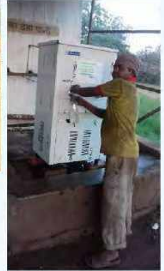
Water Cooler installed in Pellet Division
