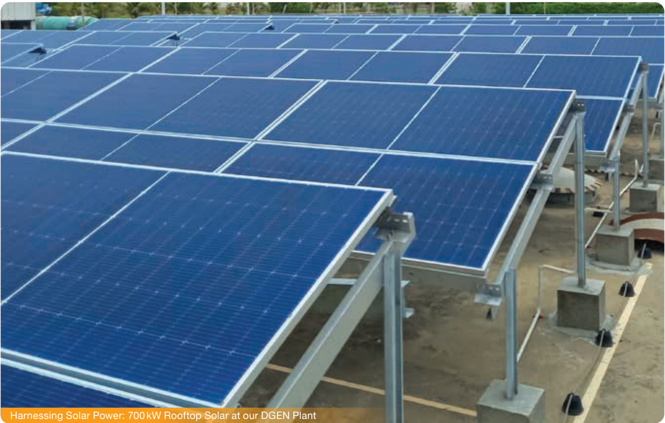
Harnessing Solar Power: 700 kW Rooftop Solar at our DGEN Plant
