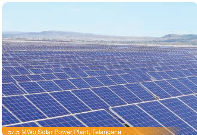
57.5 MWp Solar Power Plant, Telangana
