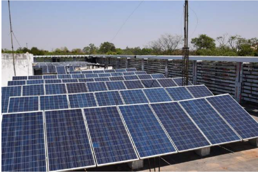
Fig. 46- Roof Top Solar Plant at CCL
