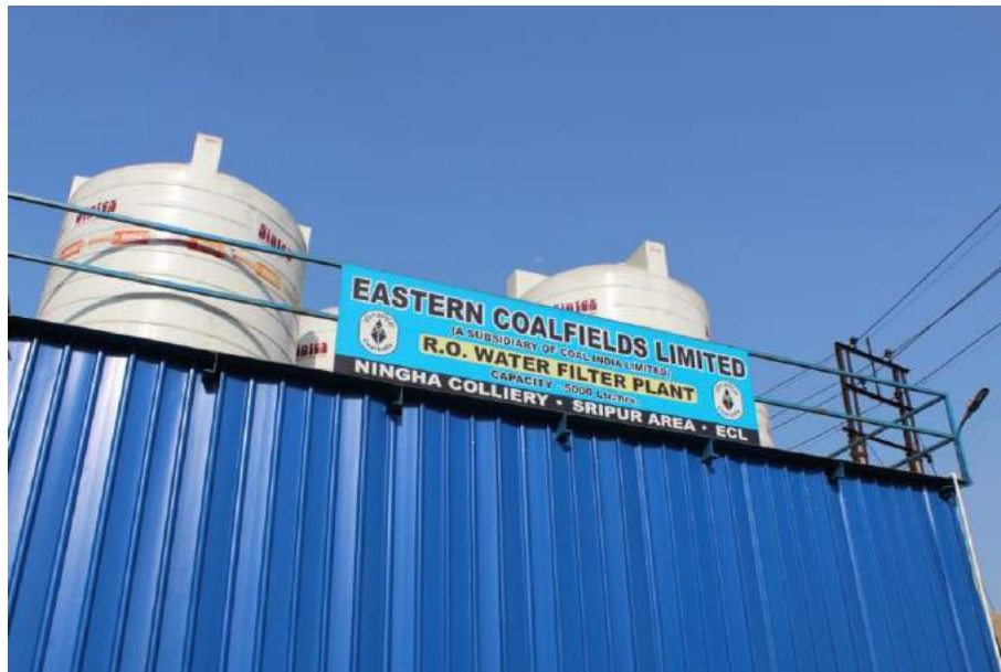
Fig. 36- R O Plant in ECL
