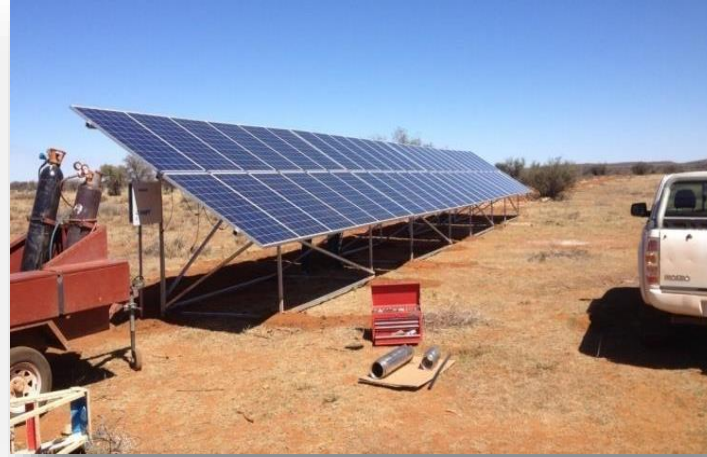
Shakti Solar Pumps Model : 10500 Watt, Discharge : 270'000 LPD (Free State, South Africa)
