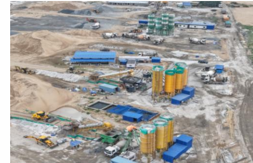
Batching Plants at Jagatsinghpur, Odisha
