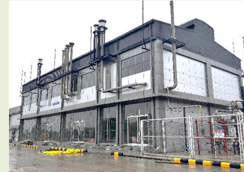
Green Hydrogen Electrolyser at Vijayanagar
