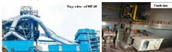
Photo: Top gas pressure Recovery Turbine installed in BF#8 at BSP
