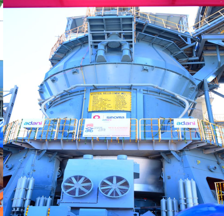
Marwar Vertical Roller Cement Mill
