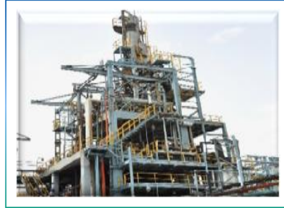
Chloromethanes plant, Mettur, Tamilnadu
