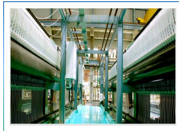
Caustic Soda manufacturing, Karaikal, Puducherry
